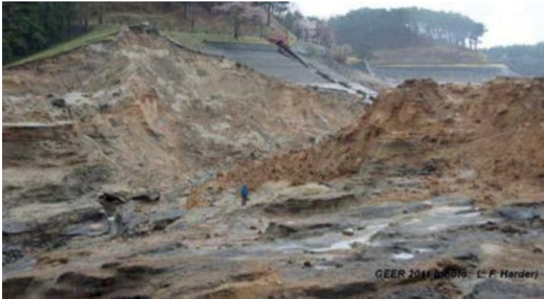
↑ Figura 7. Restos de la presa Fujinuma después del sismo de Tohoku (tomada de Preliminary Observations of the Fujinuma Dam Failure Following the March 11, 2011 Tohoku Offshore Earthquake, Japan (p. 9), por Leslie F. Harder, 2011, Geotechnical Extreme Events Reconnaissance).
